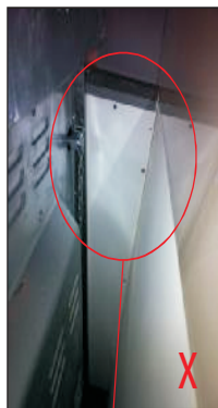
Left Side of oven, chain not attached
